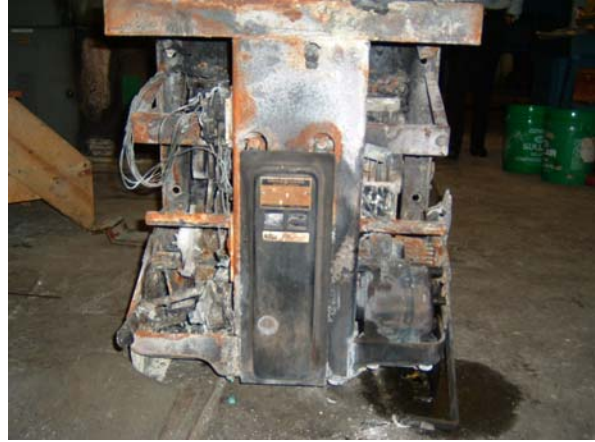
Fig. 3 Extensively Damaged Generator Breaker
