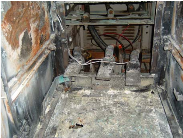
Fig. 2 Damaged Breaker Cubicle
