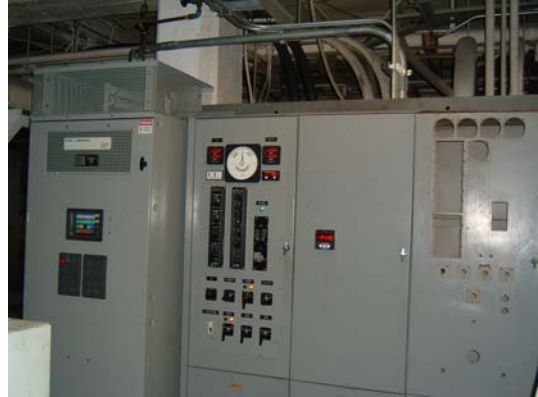
Fig. 10 Completed Retrofitted Switchgear Showing Excitation, Protection and Synchronizing Control Systems
