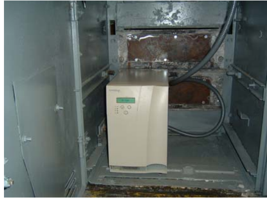
Fig. 9 UPS System Installed in Switchgear Cubicle
