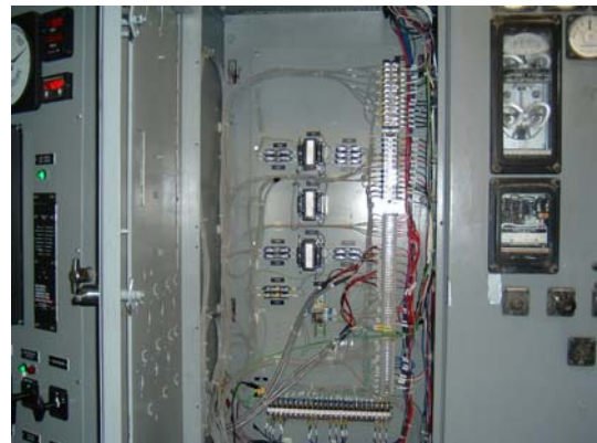
Fig. 6 Internal Sub-Panel for Protection and Control Circuits
