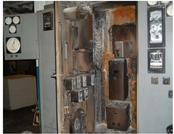
Fig. 4 Damaged Excitation Control and Synchronizing Equipment and Metering
