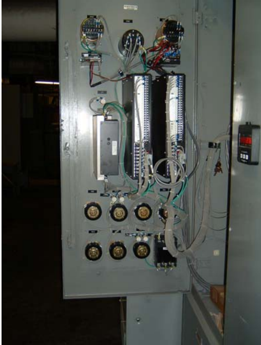
Fig. 7 Back of Protection and Synchronizing Control Sub-Panel
