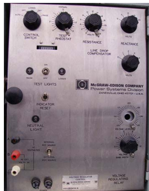
Pennsylvania McGraw-Edison Pole Star Hinge Pins on Right of Cabinet
