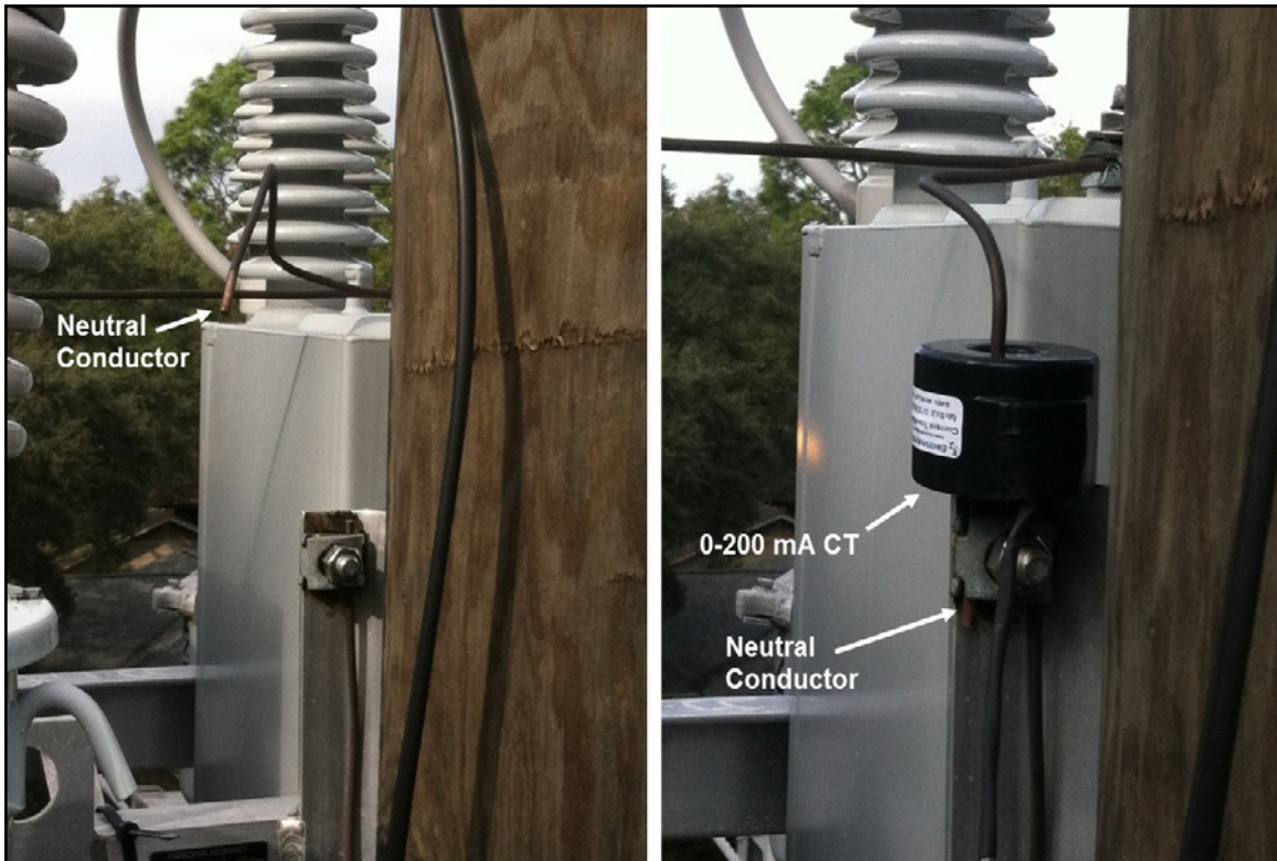
Figure 5: Neutral Current CT Installation
